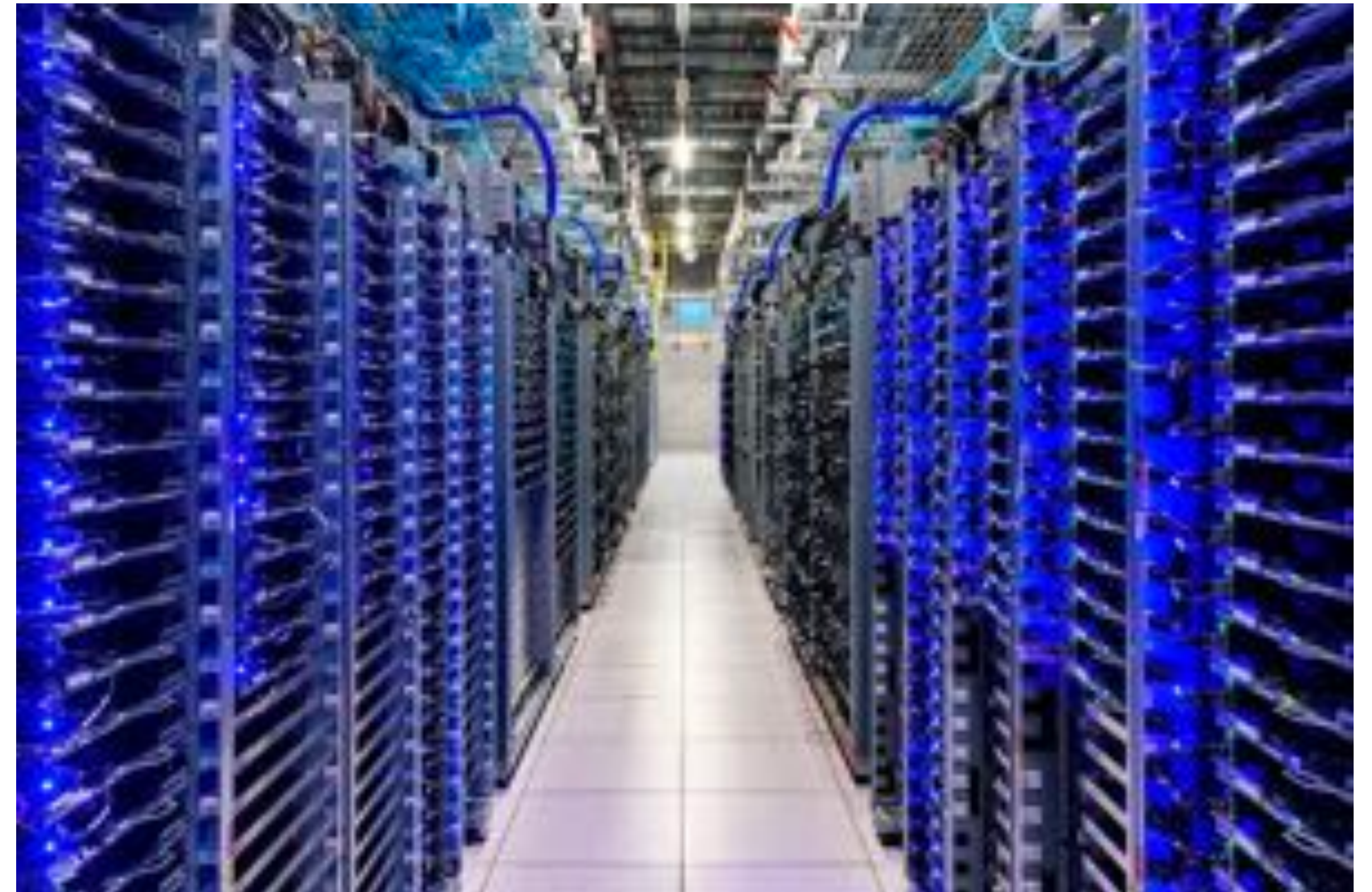
Example of a supercomputer in a Data Center
